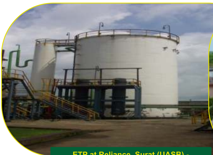
ETP at Reliance, Surat (UASB) - Gas Generation 312/M3/hr
