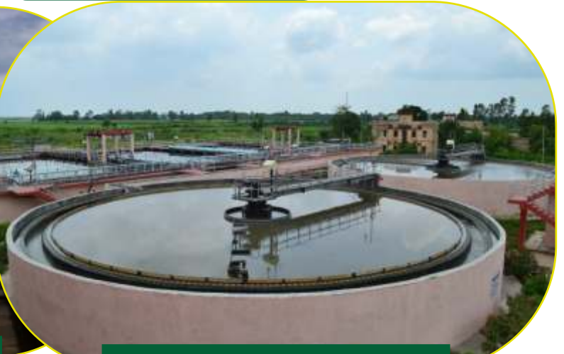
27 MLD STP at Haridwar (SBR - C TECH)
